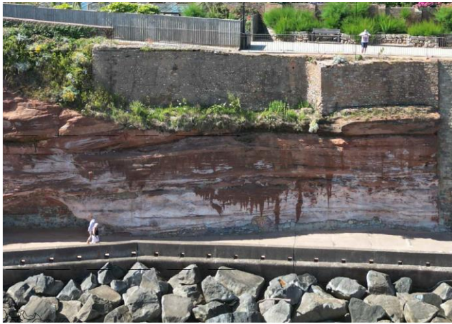
View of cobblestone retaining wall at risk of falling
